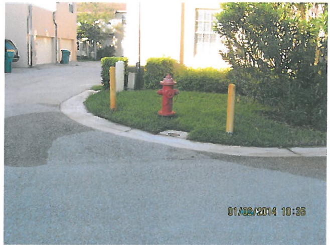
Typical Fire Hydrant
